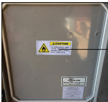
INSIDE OF ELECTRICAL BOX
